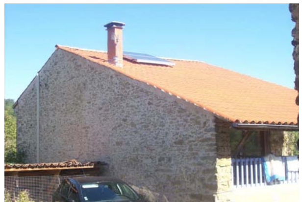
New roof and solar heating added to several hundred year old stone cottage
