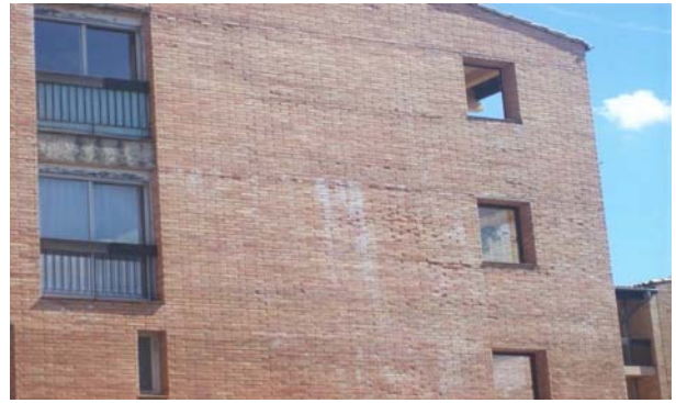
Poor quality brick work on apartment building
