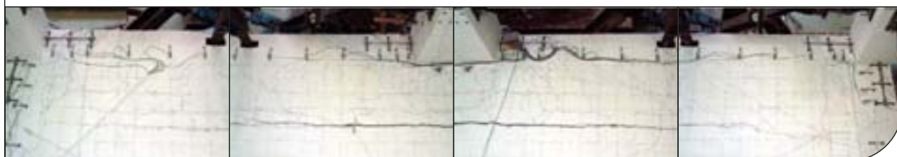
Figure 1 Separation of floor slab putting high strains on topping reinforcement. Source: University of Canterbury Civil Engineering Department, J Matthews
