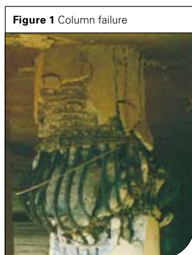
Photo courtesy of the New Zealand Society for Earthquake Engineering Reconnaissance Team Northridge 1994
