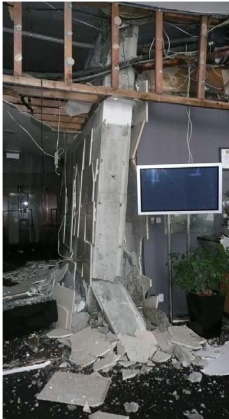
Figure 4: Shear wall D5-6 base failure (in the hotel foyer)
